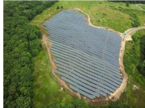
This 4.2-MW dual-use community solar project, located on a blueberry farm in Rockport, Maine, represents the fourth solar project CS Energy has executed on time and on budget for BlueWave Solar, and Navisun LLC, since 2017.
